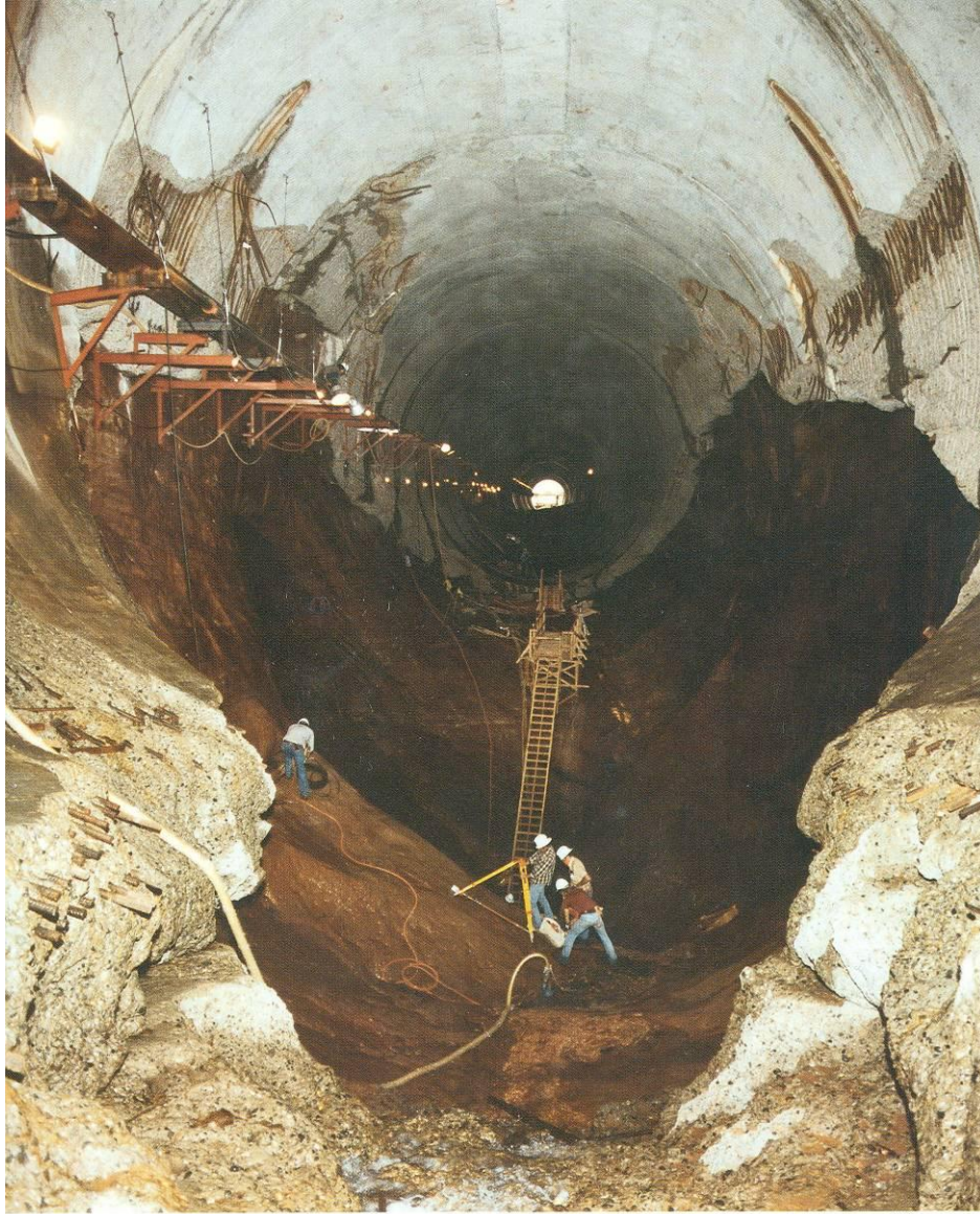
FRONTISPIECE—Glen Canyon Dam. Left Spillway Tunnel Sept. 1983. The “big hole” in the spillway invert was 11 meters deep. Photo C557-400-690NA
